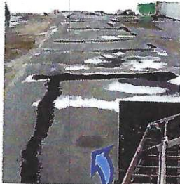
OLD PATCHED ROOF
